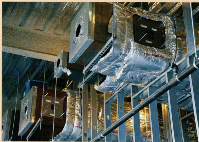
Grease ducting with ULtimate doors in place awaiting layers of high temperature insulation. Door insulation blankets are installed over long studs attached to the door.
