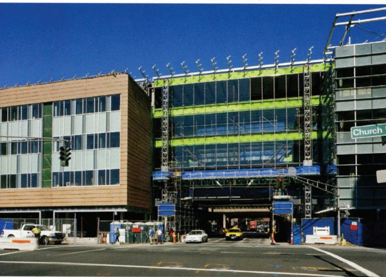
Gateway Community College's $198 million addition in downtown New Haven, Conn., is seeking certification from U.S. Green Building Council's Leadership in Energy and Environmental Design program. Images supplied by Ductmate Industries.
