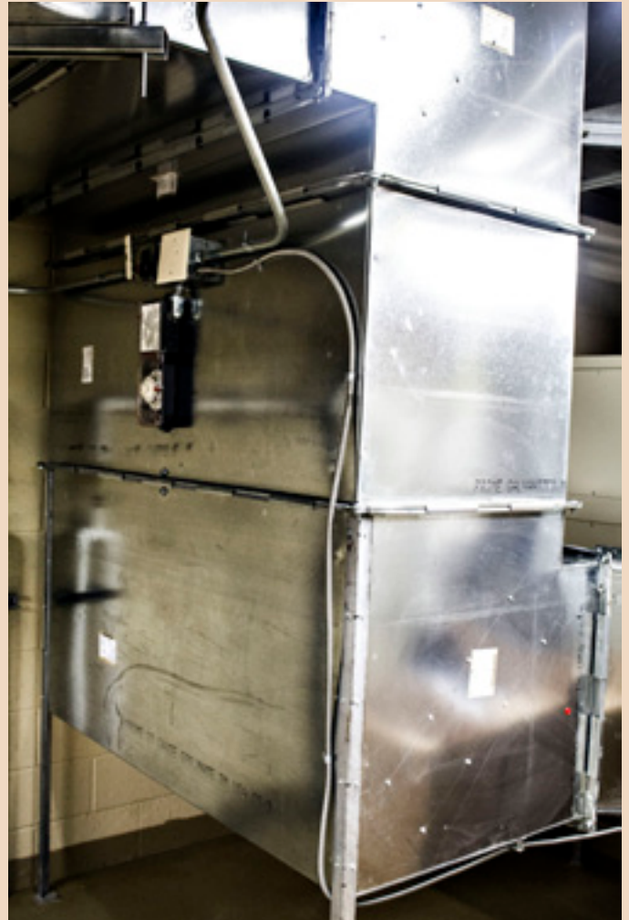
Ductwork up to 80 inches in diameter is used throughout the student housing and recreational building.
