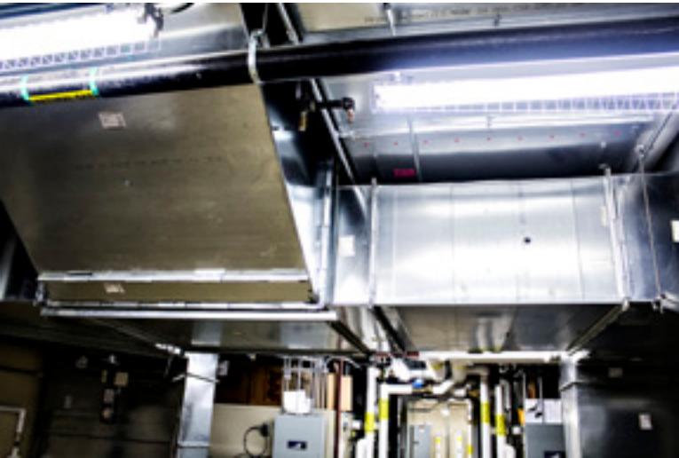
Installing PolyArmor duct liner inside the ductwork does not increase the system's weight, Ductmate officials say.
