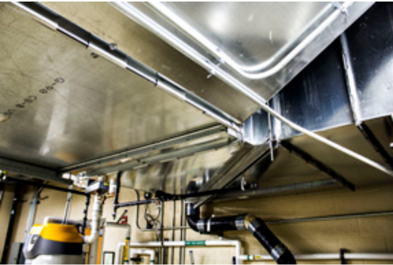
The Indiana University of Pennsylvania project uses Ductmate Industries' PolyArmor polyester duct liner on HVAC system for the residential and recreational center project.
